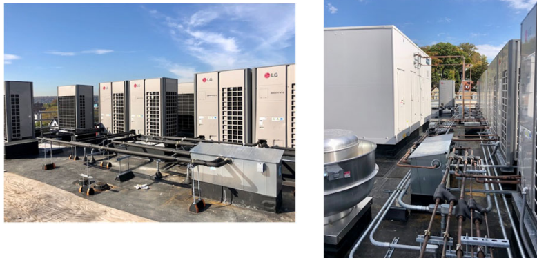
Piping rooftop ERU and HP units at Academic Building.
